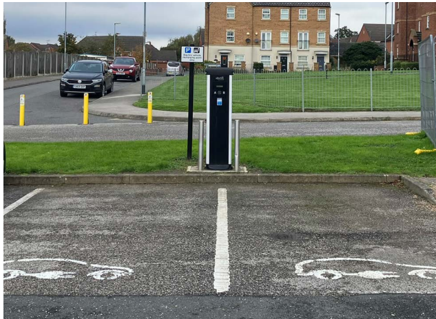
Figure 41: Public EV charging infrastructure (elsewhere in the UK).
